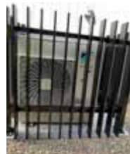
Air Conditioner Condenser Unit
