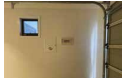
Location of the Switchboard.
